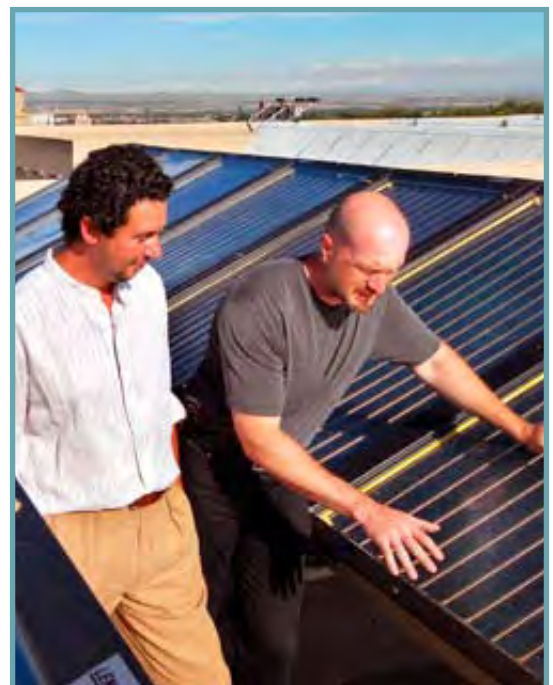
UNM professors Andrea Mammoli (left) and Peter Vorobieff examine solar thermal collectors on the roof of the Mechanical Engineering Building on the UNM campus. Sandia is helping upgrade the solar system to the latest technologies.
